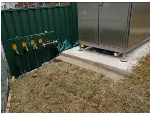
Figure B.8 Installation of sampling taps for raw water and various stages of filtered water
