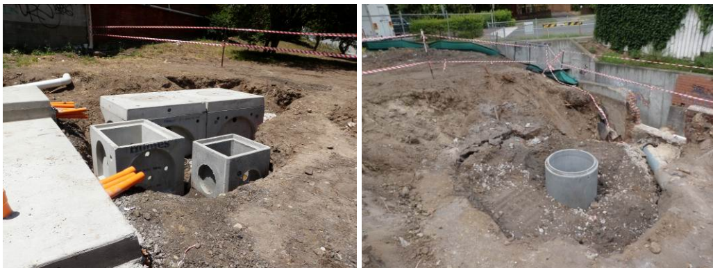
Figure B.4 Installation of product water, control valve and return pits and sump pit
