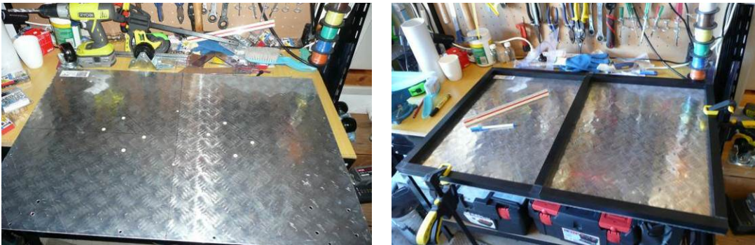
Figure 3.12 Construction of filter column filtration system – Constructing and reinforcing the base plate for stability
