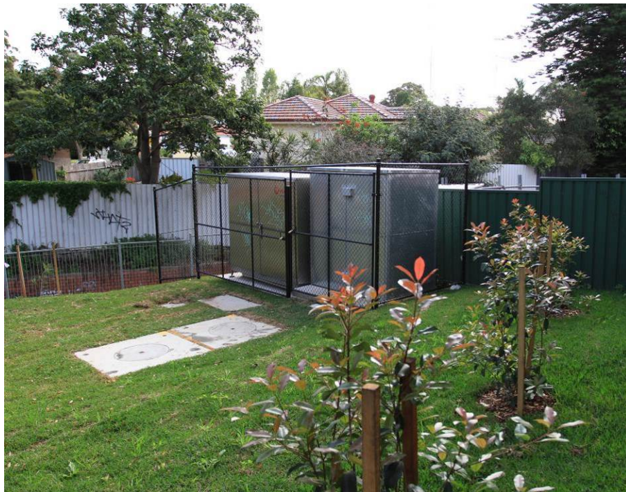
Figure B.9 Completed Harvesting Plant with security fencing and re-vegetation of site
