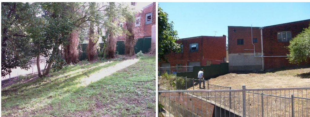
Figure B.1 Lower West Street Reserve, Carlton before commencement of works & clearing of trees
