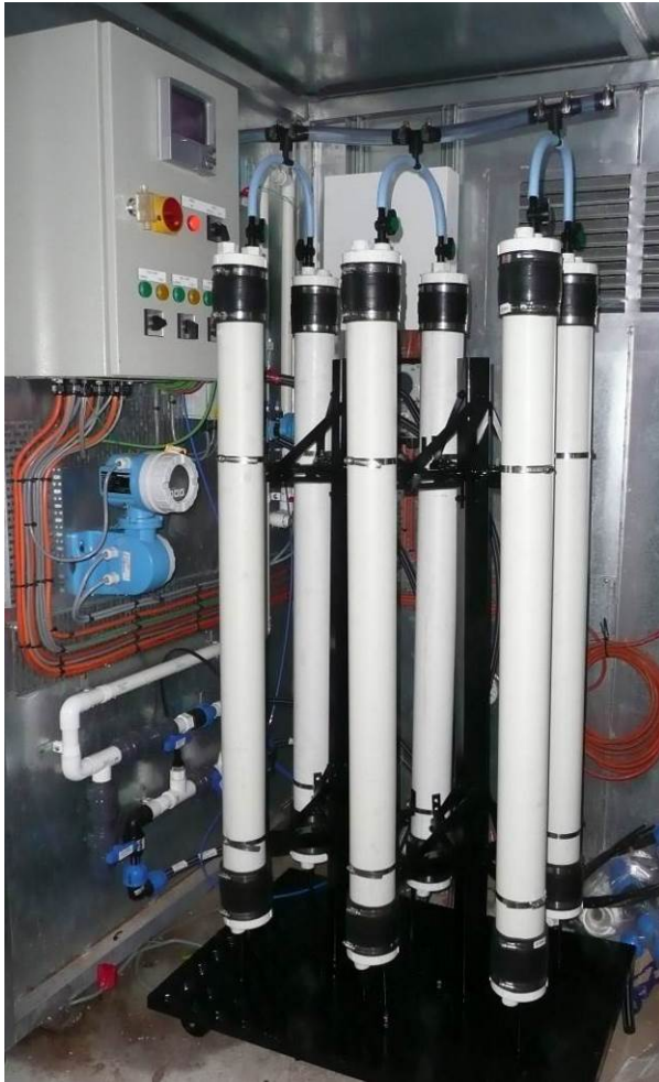
Figure 3.16 Filter column filtration system in stormwater harvesting plant cabinet
