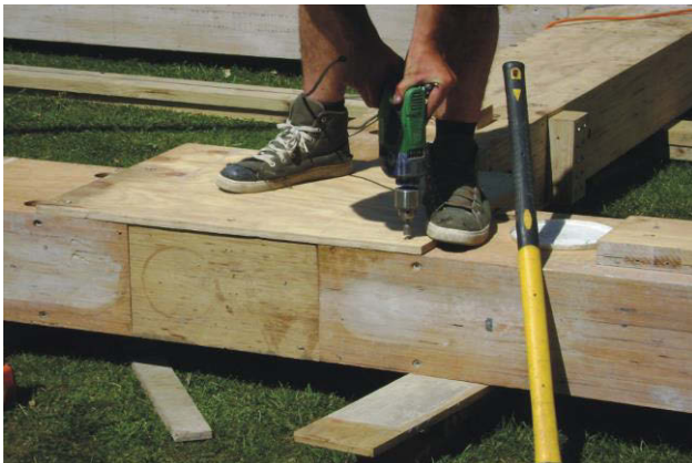
Figure 8.8 Temporary plywood gussets (non-engineered)
