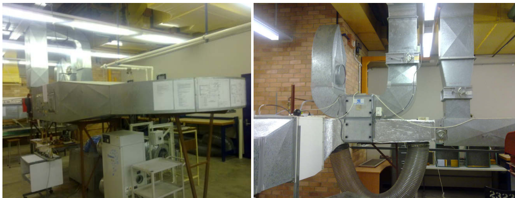
Figure 6.15 Air Handling Unit (AHU) of UTS laboratory
