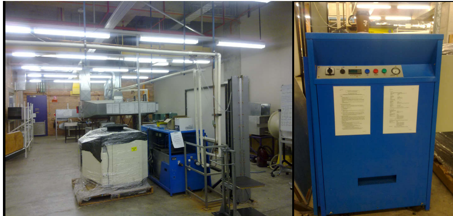
Figure 6.14 Chiller and cold water system of HVAC lab.
