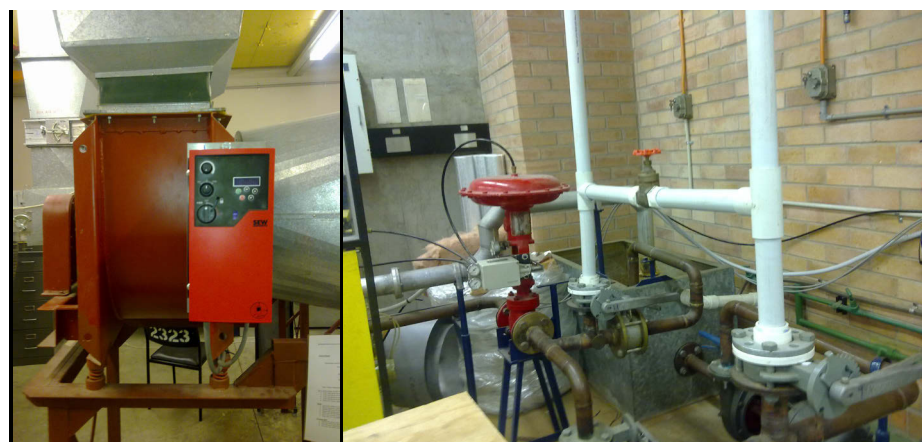
Figure 6.12 actuators system for UTS HVAC room temperature control
