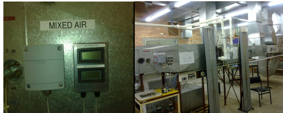
Figure 6.11 Measurement systems for HVAC laboratory of UTS
