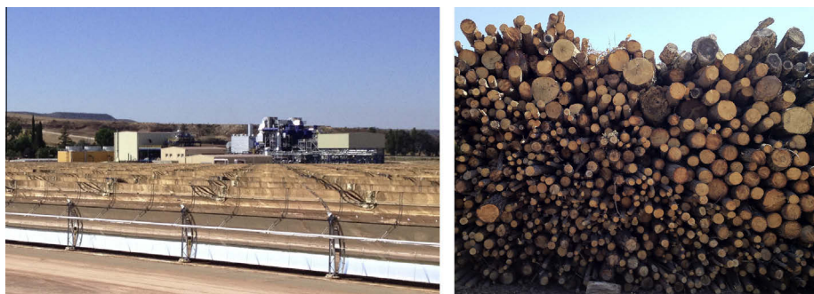
Fig. 1. First CSP-biomass plant under construction near Lleida, Spain (left) and its biomass fuel (right).
