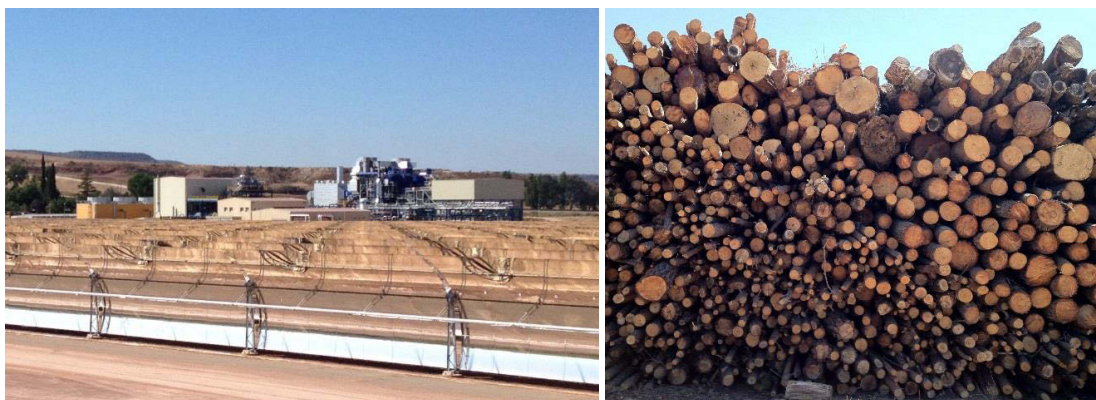
Figure 1: First CSP-biomass plant under construction near Lleida, Spain (left) and biomass fuel (right)
