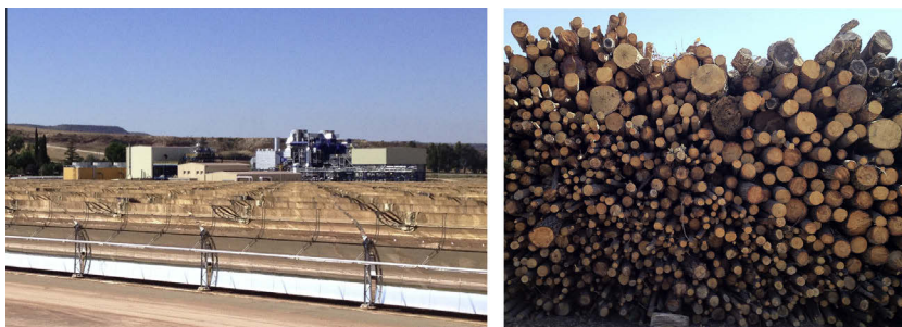
Fig. 1. First CSP–biomass plant under construction near Lleida, Spain (left) and biomass fuel (right).
