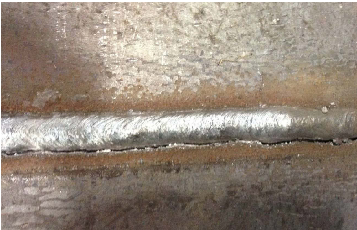
Figure 4-9: Fully developed fatigue crack along the weld toe.
