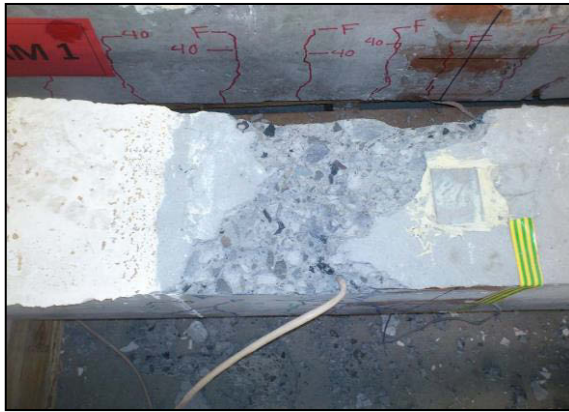
(a) Loose debris removed from the top
