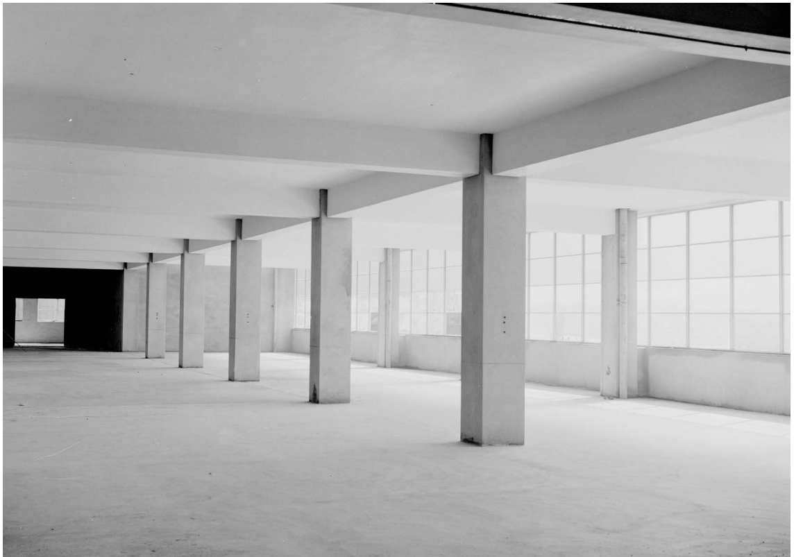
Fig. 27 The third floor interior of the new Government Printing Office building in Ultimo, 1957, pared back and distinctly modern, before the electrical fittings, plumbing and flooring were installed. Note the necessity for columns; the building was not clear-span owing to the lack of steel production in the 1940s and early 1950s. Copyright of the Crown, reproduced with permission, courtesy of the Mitchell Library, State Library of New South Wales, Sydney. SLNSW call no. Government Printing Office 2 – 08786. Reproduced in the publication New Government Printing Office (1957).
