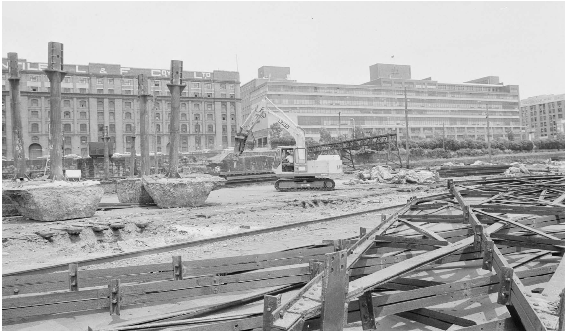
Fig. 11 Demolition and rebuilding of Darling Harbour with the Government Printing Office in the background (right), 1985. Copyright of the Crown, reproduced with permission, courtesy of the Mitchell Library, State Library of New South Wales, Sydney. SLNSW call no. Government Printing Office 4 – 36990.
