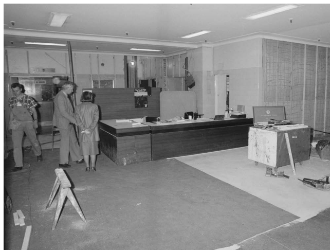
Fig. 99 Renovations to the front entrance and foyer, 1986. Copyright of the Crown, reproduced with permission, courtesy of the Mitchell Library, State Library of New South Wales, Sydney. SLNSW call no. Government Printing Office 4 – 44277.
