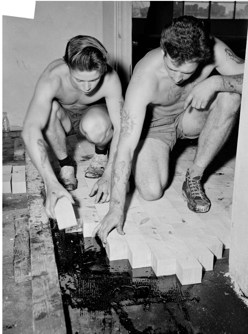
Fig. 46 John Lumley (right) and another worker lay the woodblock floors at the Government Printing Office, c. 1958. Courtesy of the Mitchell Library, State Library of New South Wales, Sydney. SLNSW call no. Government Printing Office 2 – 16673.
