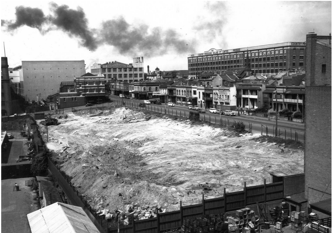
Fig. 33 Site preparation for the new Government Printing Office building, Ultimo, 1951. Courtesy of the Mitchell Library, State Library of New South Wales, Sydney. SLNSW call no. Government Printing Office 1 – 07712. With thanks to Geoff Hawes for the print.
