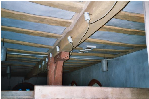
Figure 11 Timber ceiling of a historic church showing signs of over-loading
