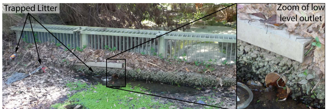
Figure 1-5 – Trash rack GPT, with trapped leaf litter and low flow outlet.
