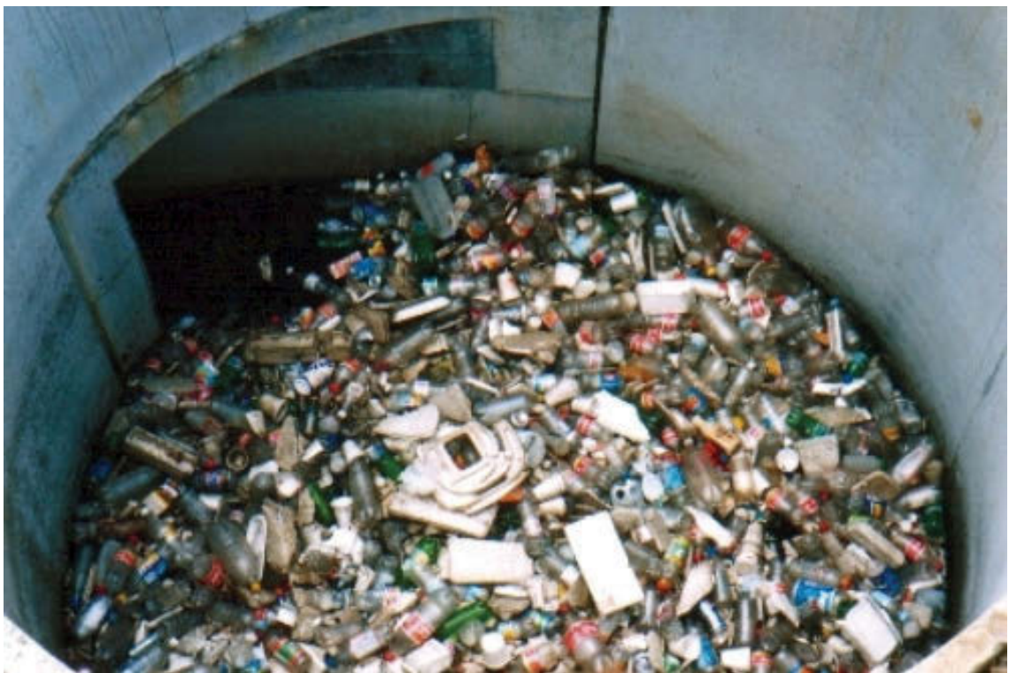
Figure 1-3 – Photograph of the full sump of a continuous deflection device prior to cleaning (Rocla, 2009).
