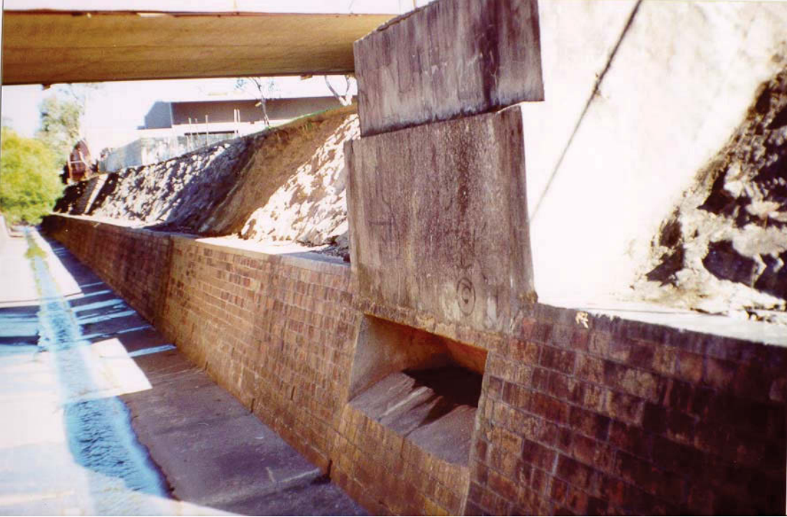
Figure 1-6 – A photograph of sewer overflow structure in Sydney that is designed to discharge effluent directly into a concrete lined stormwater channel near Punchbowl (Avis, 2001).
