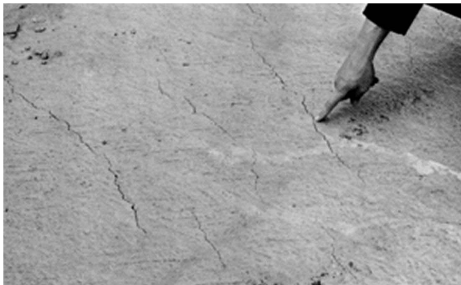
Figure 2.13: Plastic shrinkage cracking, a typical defect of pavement slabs (PCA 2001)
