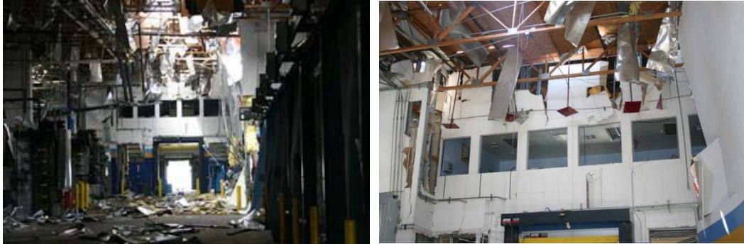
Figure 3.3: Ethylene oxide sterilization facility damage
