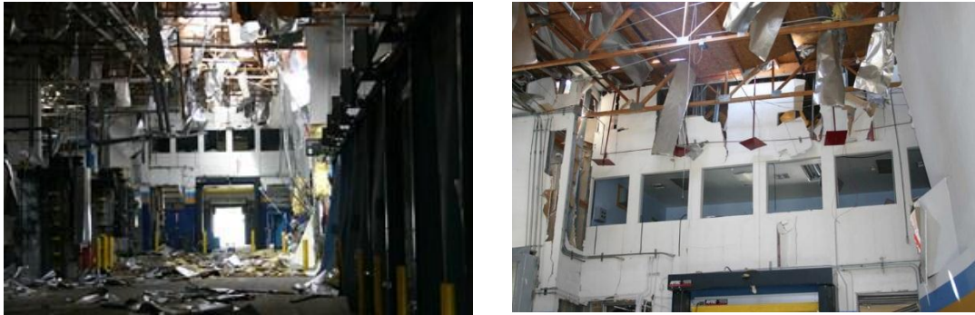
Figure 4: Facility damage (CSB, 2006).
