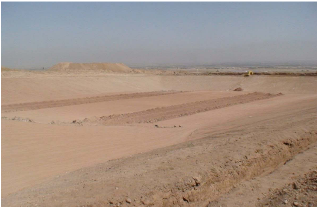
Figure 7.6: Excavation for Leachate Collection System of Tehran Sanitary Landfill (Photo Taken by the Author)
