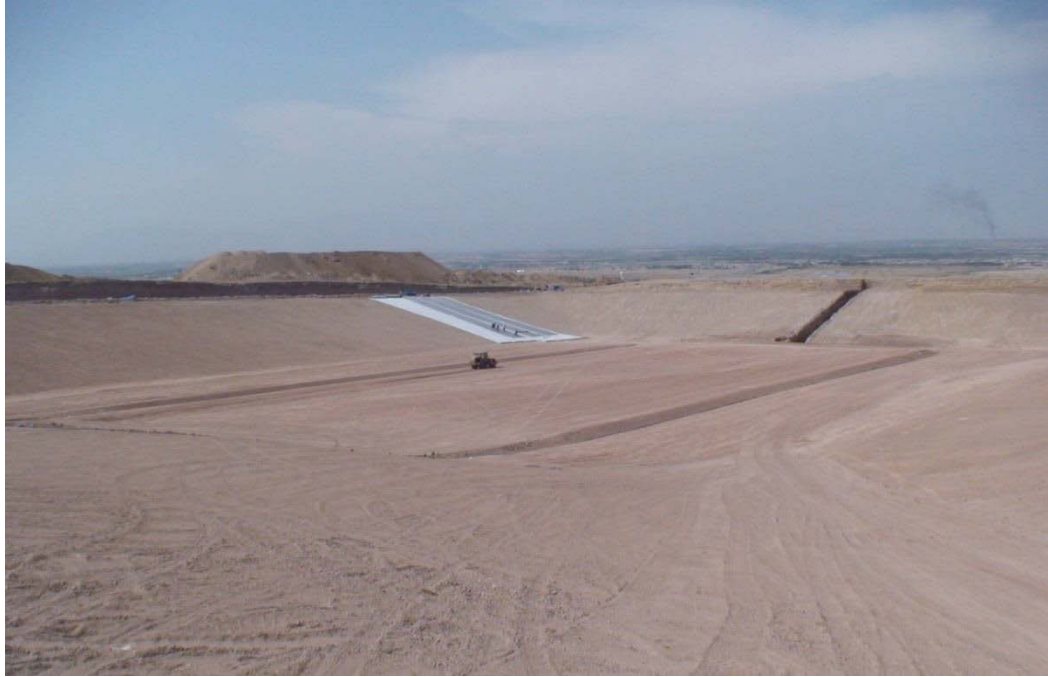
Figure 7.7: Covering Tehran Sanitary Landfill with Geosynthetic Base Liners (Photo Taken by the Author)
