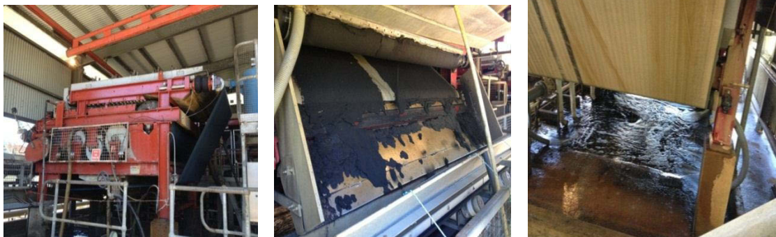
Figure A-3 Belt filter presses at St. Marys WWTP
