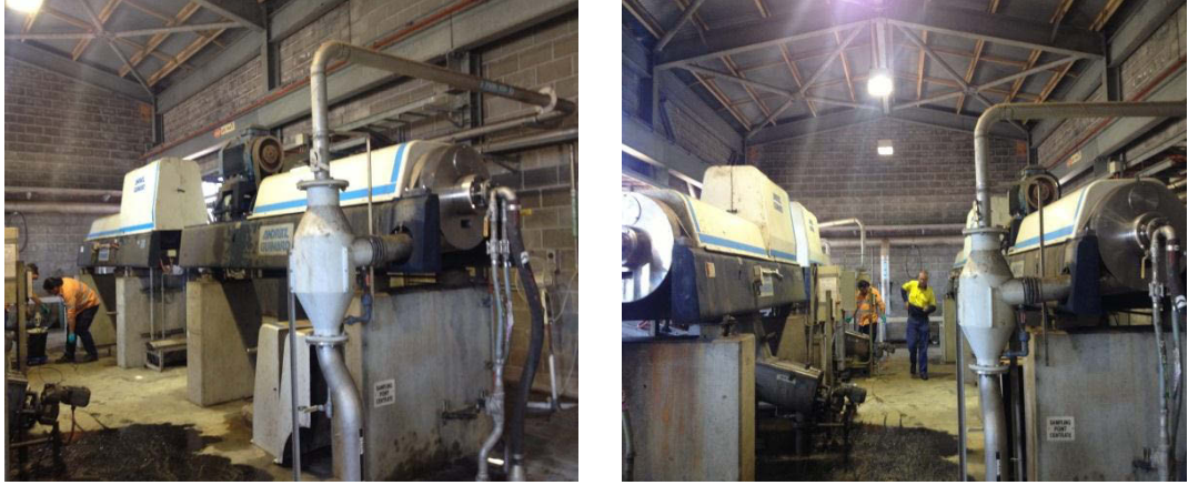
Figure A-1 Centrifuges at Wollongong WWTP
