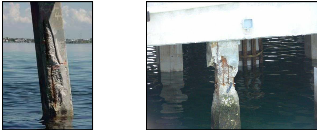
Figure 2-4 Severe corrosion in tidal zone
