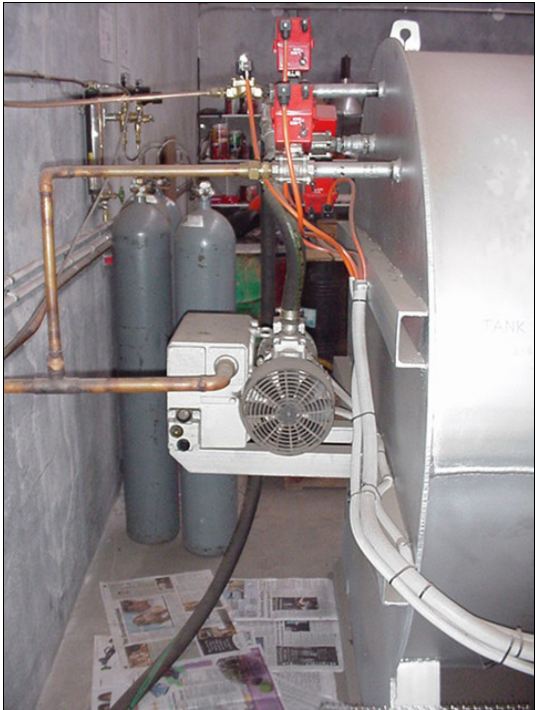
Figure 3.23: View of vacuum pump and isolation valves for hot wall vacuum furnace
