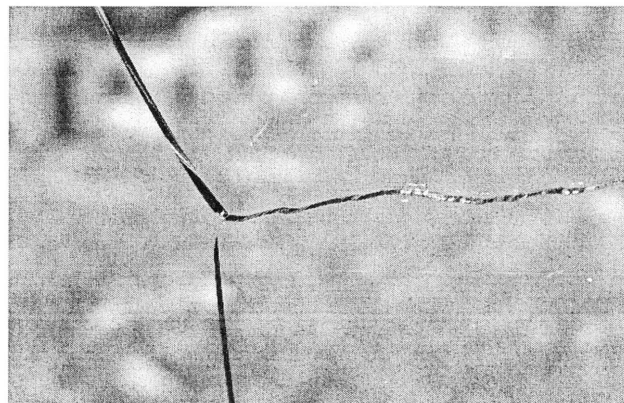
Figure 31. Cracking observed in laminated glass door of XL121 that included an absorptive solar film in its structure.
