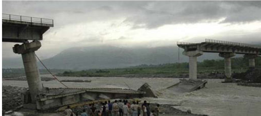
Figure 1.3 A bridge over the Gaula river in India washed away by flood in July 2008, (Bhatia (2013))
