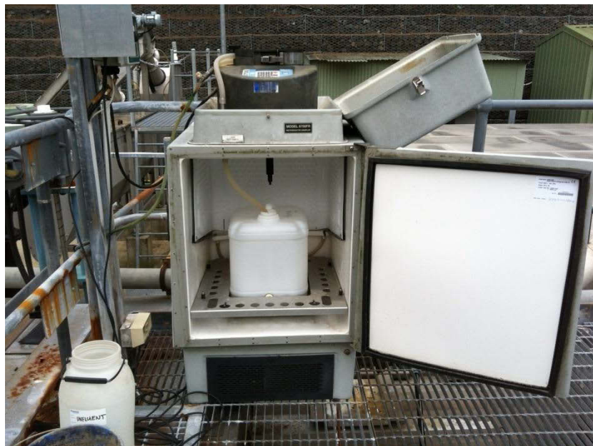
Figure 3.2 Collecting raw municipal wastewater at Sydney Olympic Park Wastewater Treatment Plant using a refrigerated sampler
