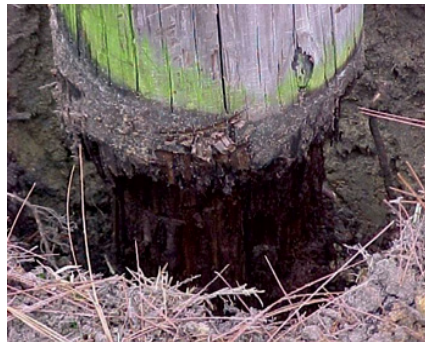
Fig. 2 Typical example of external ground line decay
