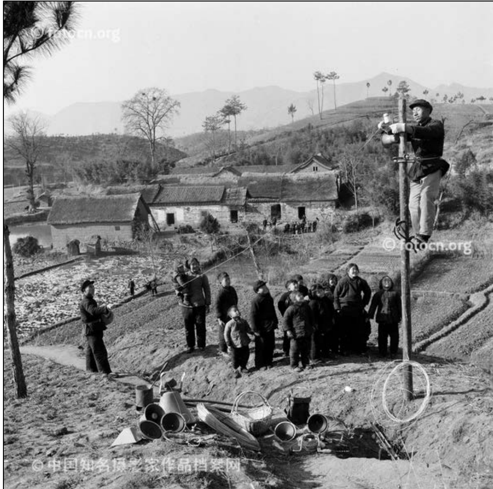
Figure 2.2 A loudspeaker being installed in Jinzhai county in 1974, in Anhui Province in Central China
