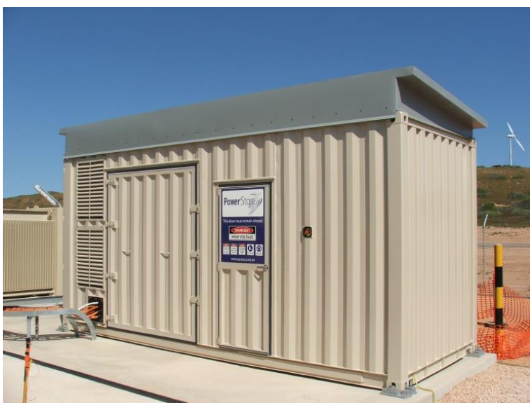
Figure 9 – PowerStore flywheel at Coral Bay, Western Australia
