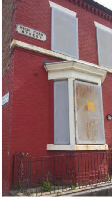
188 High Park St, Toxteth Park, Liverpool, in 2015. The whole row of houses has been scheduled for demolition
