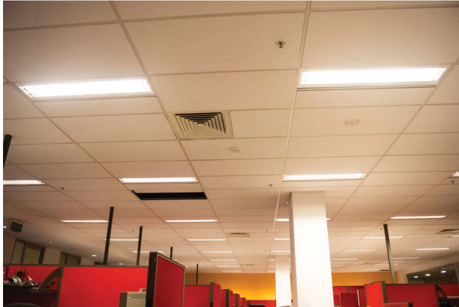
FIGURE 3.15: Planar ceiling at the Centre for Autonomous Systems(CAS), University of Technology, Sydney(UTS)
