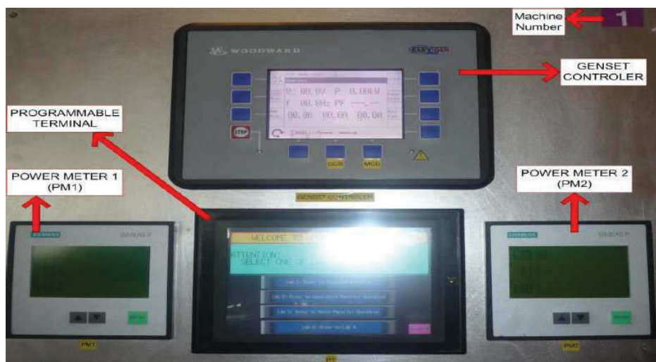
Fig. 5.16 Display and control panels of Easygen-3000 in the laboratory
